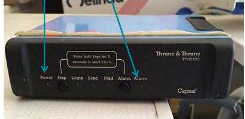
3020C "black box" (in wheelhouse) Power On & status lights
